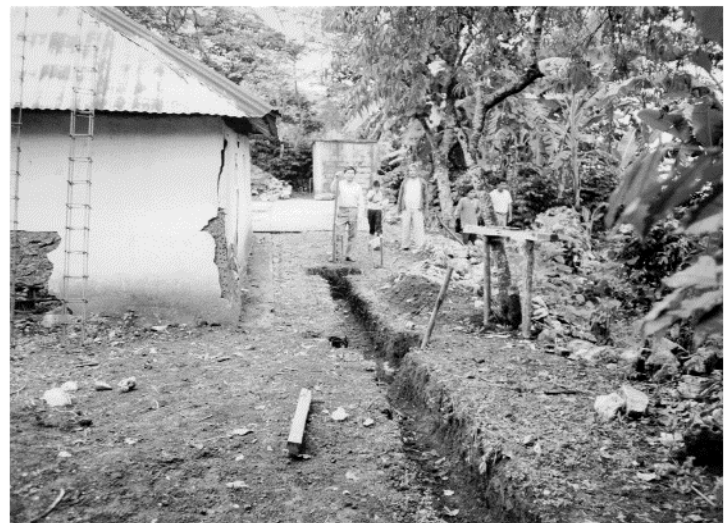
The new church will be built around the old, crumbling church, and will be exactly twice the size.
