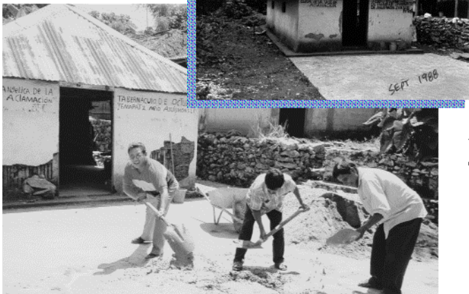
Brother Murillo and Brother Felipe (right) mix concrete for the footings.(inset) The church in '88
